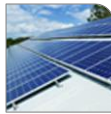
Roof Top Solar
